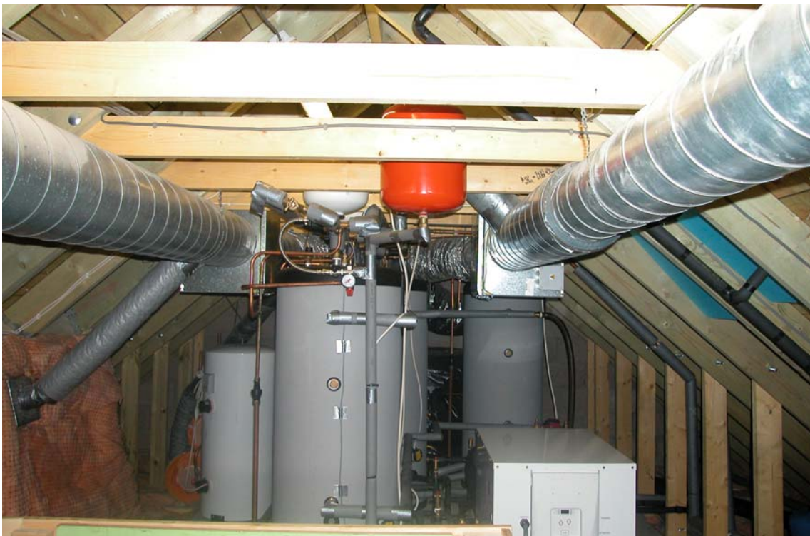
Image 9: Ducting for HRC system in loft space, sequenced hot water cylinders and heat pump (in centre of image)
