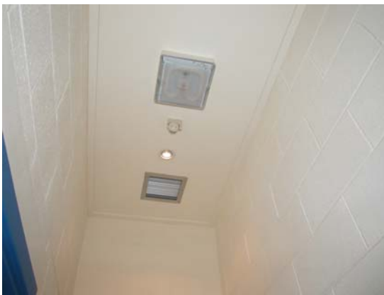
Image 8: Low-energy lighting in corridor with PIR detector
